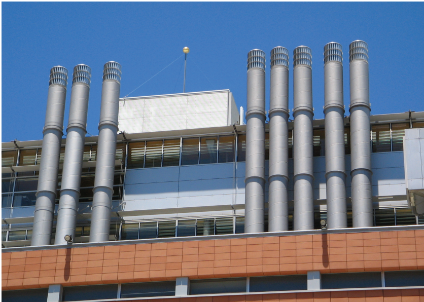
Fig. 3. Cylindrical centrifugal ventilator at the University of New South Wales
